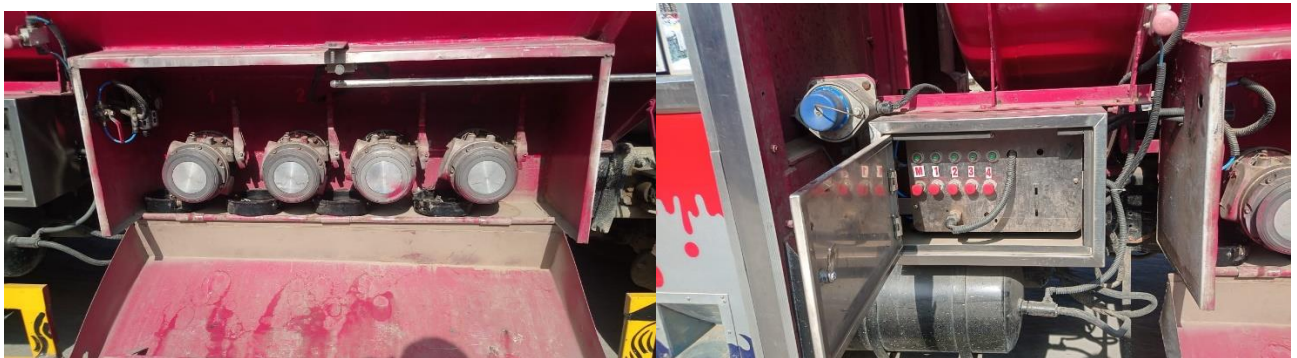
Some pictures of bottom loading ( from Thankot depot)
